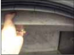
Tilt Baffle downward toward the front of fireplace
